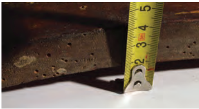
▼ Fig. 4. Lacuna in the crossbar produced as a result of the weakening of the wood due to xylophagous insects.
